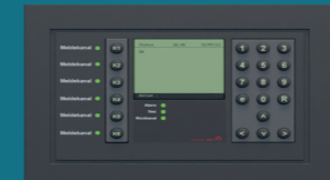
Fire alarm system (FAS)
